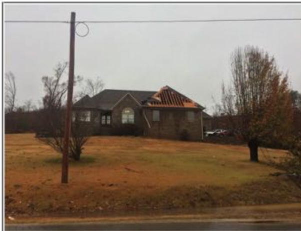
This home off of Cherokee Valley Rd sustained the most significant damage with a portion of the garage roof being removed and the garage doors being blown inward.
