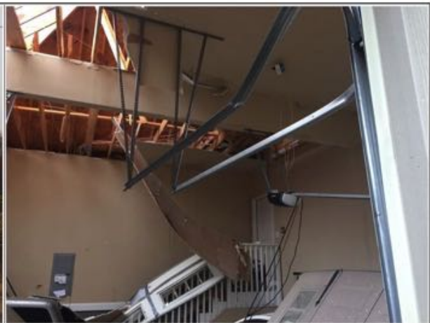
Here is the interior of the garage with the garage doors blown into the garage and part of the roof removed.
