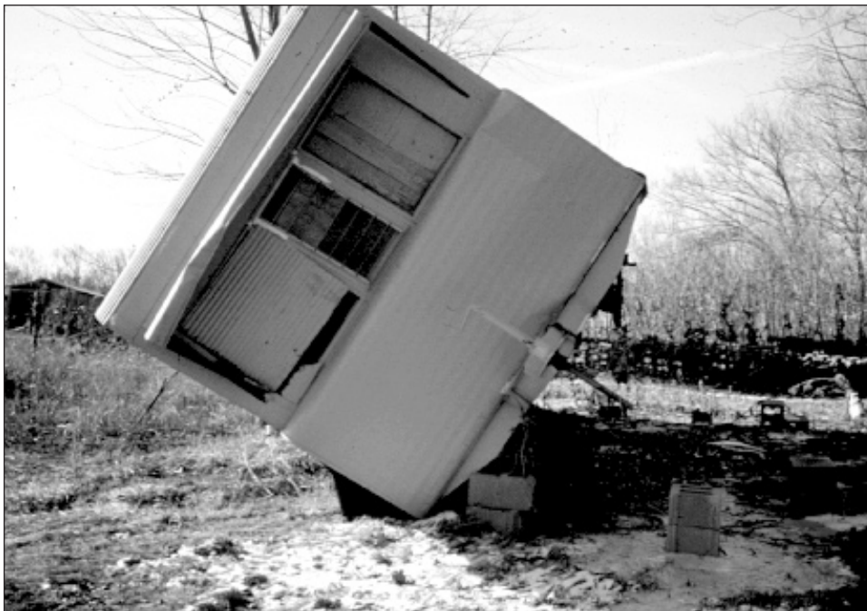
Figure 7-8. Failed foundation system that used masonry piers.
