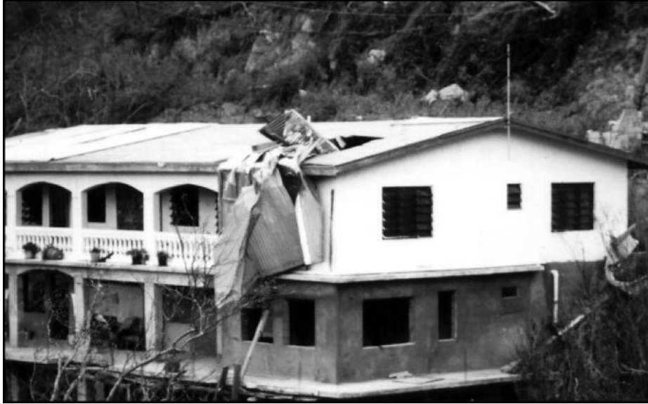
Figure 23. Hurricane Marilyn (1995). The roof of this house was penetrated by a large wind-driven missile (metal roof covering).
