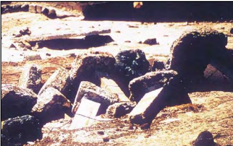
Figure 30. Hurricane Iniki (1992). Undermining of shallow footings supporting columns at Poipu Beach due to lack of sufficient embedment below erosion level.
