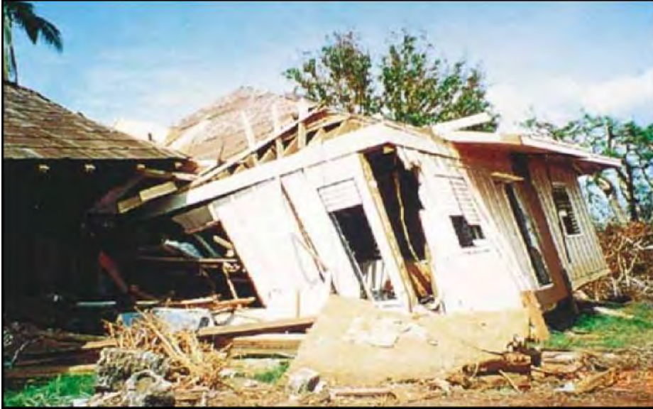
Figure 29. Hurricane Iniki (1992). Non-elevated house at Poipu Beach that floated off its foundation and was pinned against another house and destroyed by waves.
