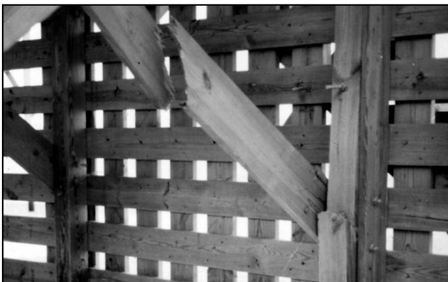
Figure 7. March 1989 nor'easter. Failure of cross-bracing.
