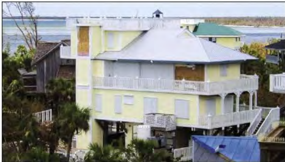
Figure 15. No structural damage was observed to homes built to the 2001 FBC (North Captiva Island, FL, 2004).
