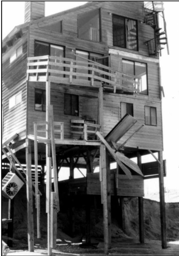
Figure 6. March 1989 nor'easter. Although this house seems only to have lost decks and a porch, the loss of supporting soil compromises its structural integrity.
