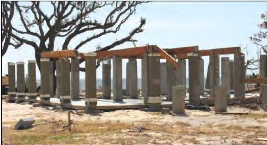
Figure 21. This elevated house on a masonry pier foundation was lost, probably due to waves and storm surge overtopping the foundation (Long Beach, MS, 2005).
