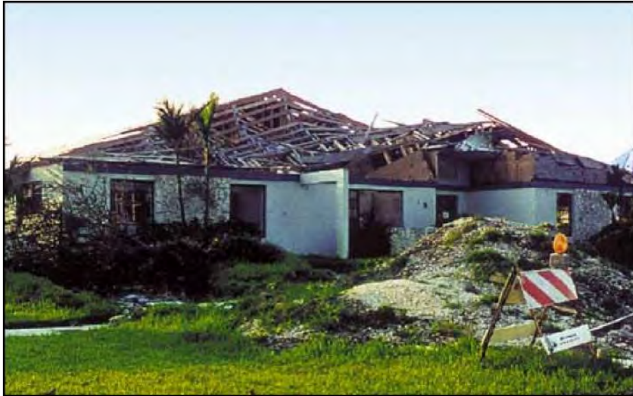
Figure 13. Hurricane Andrew (1992). Roof failure due to inadequate bracing.
