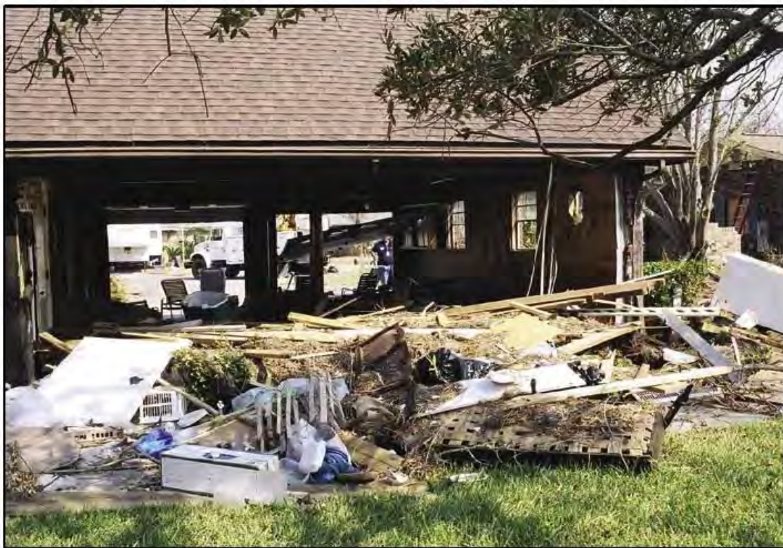
Figure 20. This house, located in Zone AE, experienced Zone V surge and wave conditions (Santa Rosa Sound, FL, 2004).
