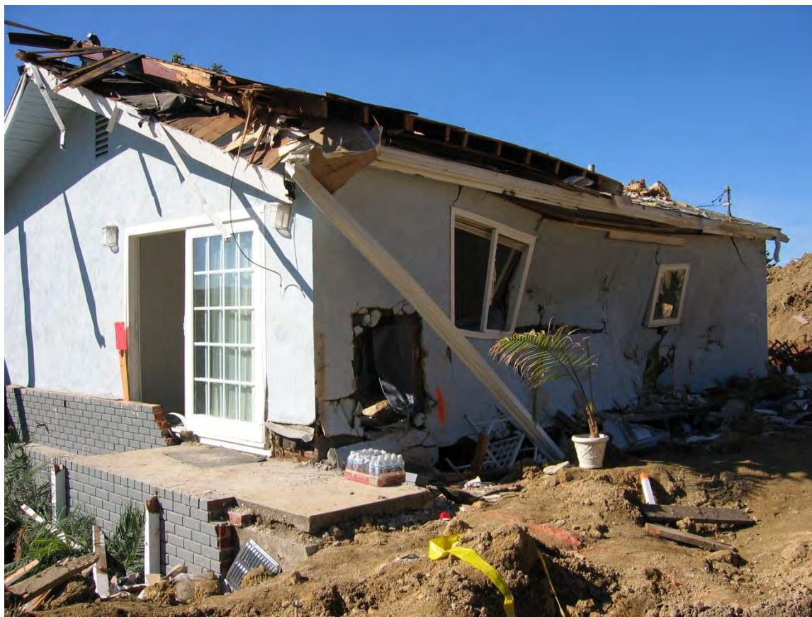
Figure 28. Damaged building braced for structural support in La Conchita, CA, after January 2005 storm event.
